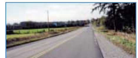
Rt. 12, Owen Sound, Ontario, paved with TOR plus GTR shows no cracks after 2 1/2 years.
