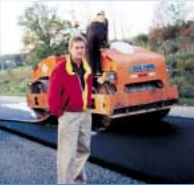
Rolling was begun immediately after laying the mix – with no adhesion to the rollers
