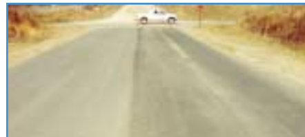
5202 St, Lincoln, Nebraska. Left side, paved with standard mix depicts stripping of asphalt. Right side, with TOR plus GTR with no stripping after 1 1/2 years.
