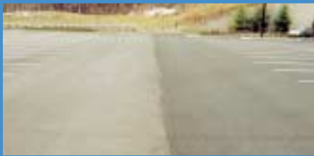
Degussa Headquarters parking lot, Parsippany, New Jersey. Left side, standard asphalt. Right side, TOR plus GTR after 2 years.
